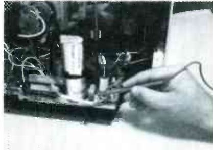
PROBING THE SHADOWY AREAS near the flyback revealed a cracked resistor. It proved to be the cause of the mysterious streaking.
